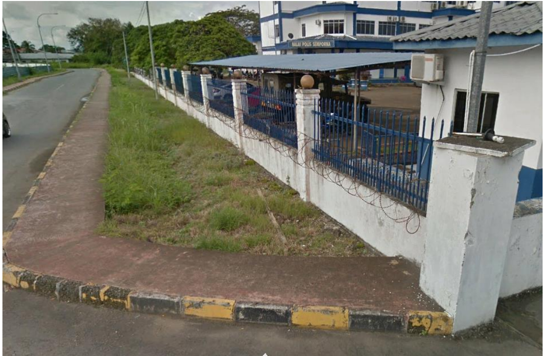
Photo 3.8 Picture of earth drain located in front of Police Headquarters along with Jalan Balai Polis
