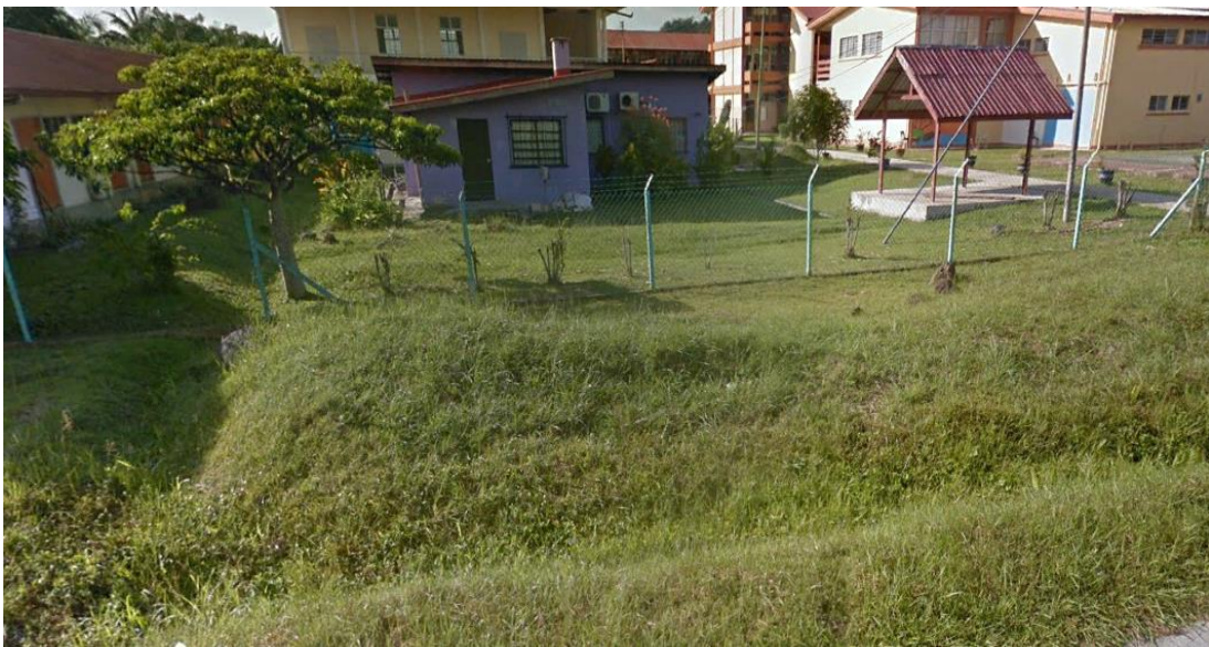
Photo 3.11 Picture of earth drain in front of SMK Datuk Pg. Abdullah along Jalan Balung-Semporna
