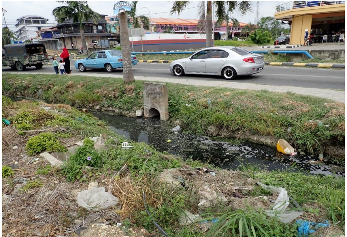
Photo 3.2 Example of earth drain located within the study area (Earth drain along with Jalan Hospital, facing downstream)
